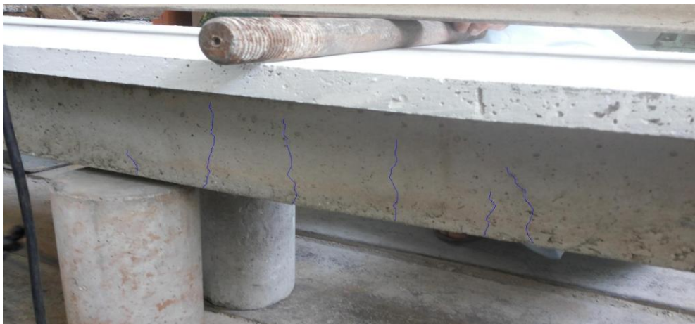
Figure 10: Cracks pattern under loading
