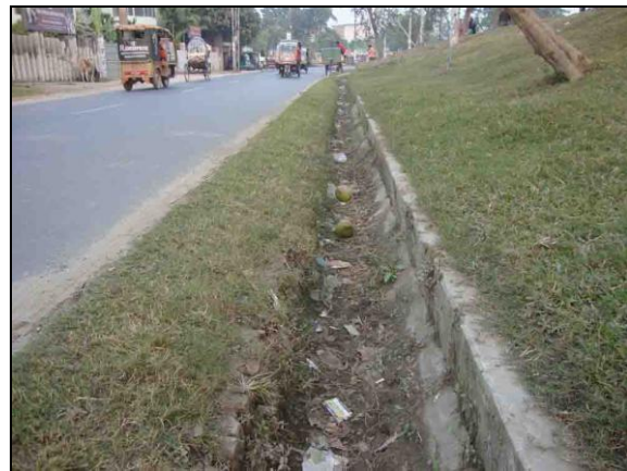
Figure 5: Road side drain blocked by bushes & sharbs near Hadir Mor
