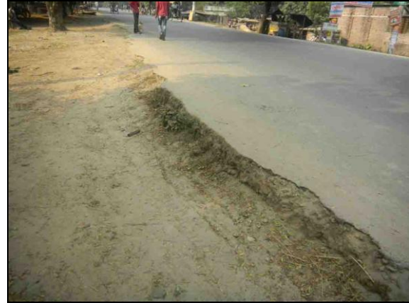
Figure 4: Inadequate drainage facilities cause serious deterioration of the pavement by continuous soil erosion at Katakhal
