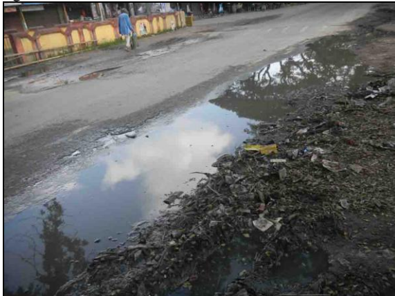
Figure 3: Soil stabilities gradually decrease due to long term water logging situation at Naudapara Bazar
