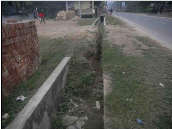
Figure 6: Drainage is blocked by dumping of soil beside Vodra to Meher Chandi road
